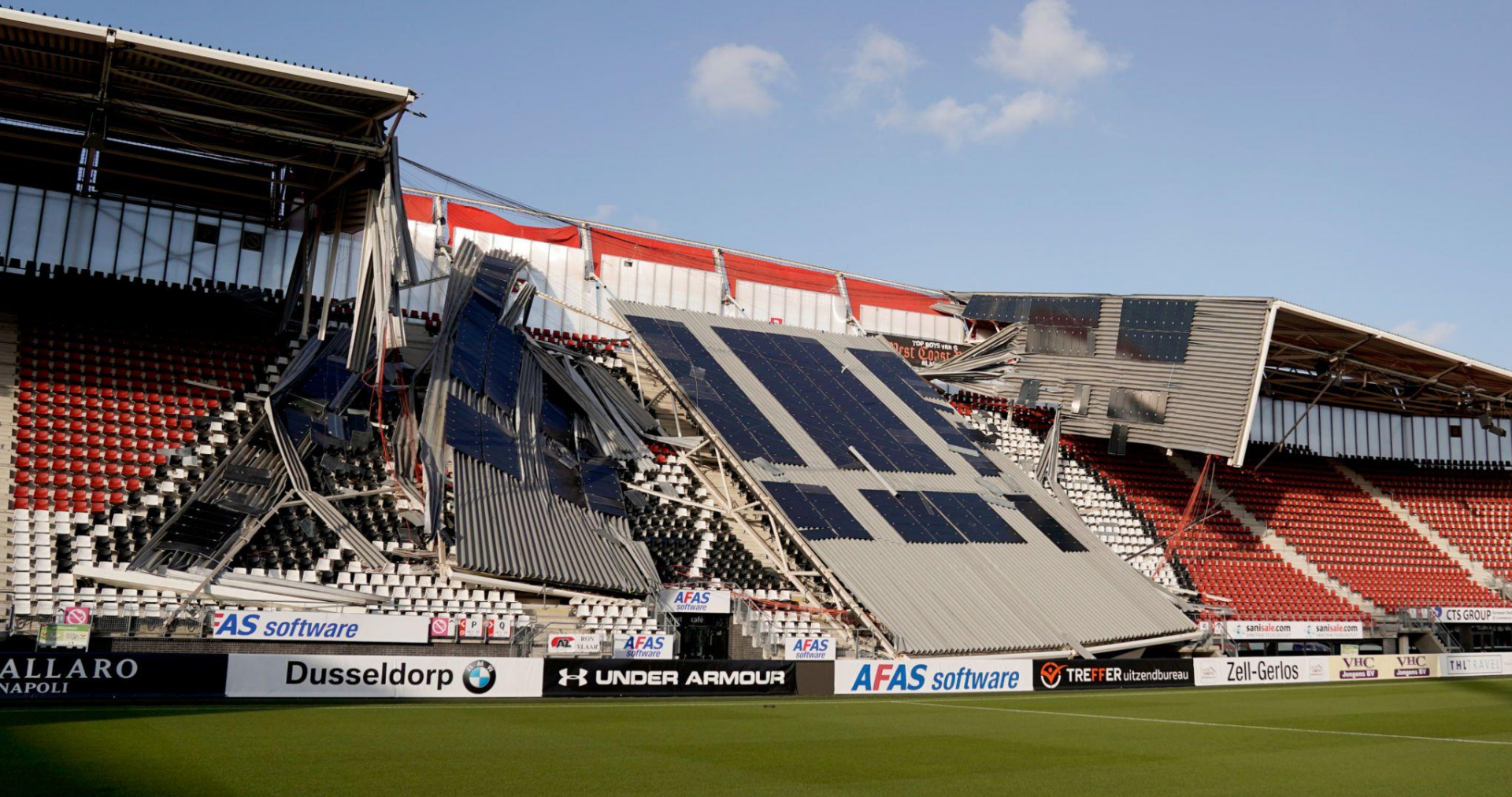
Alkmaar (NL) stadium roof damaged during storm 10 August, 2019
